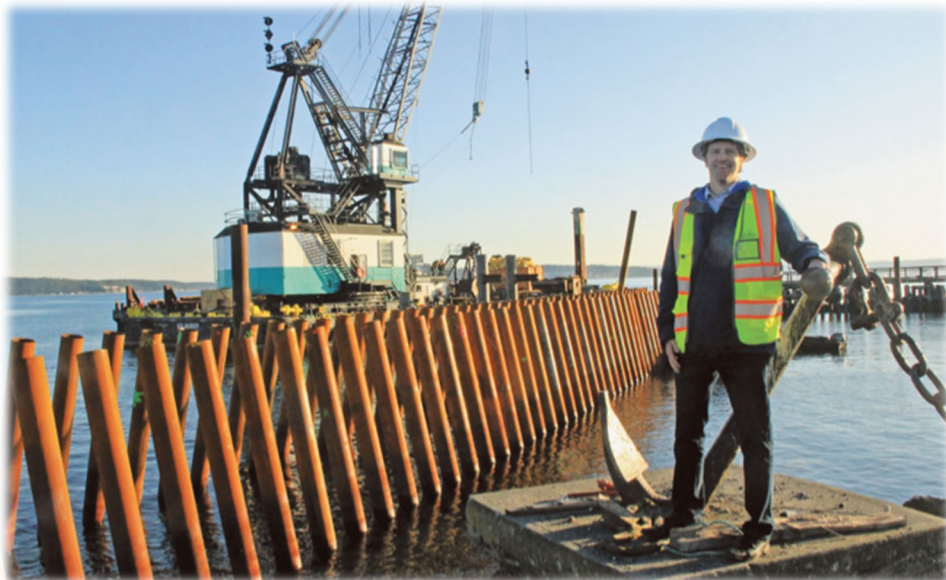
Image: Port Engineer Matt Klontz Oversees Reconstruction of the Point Hudson Jetty – Summer 2023.
