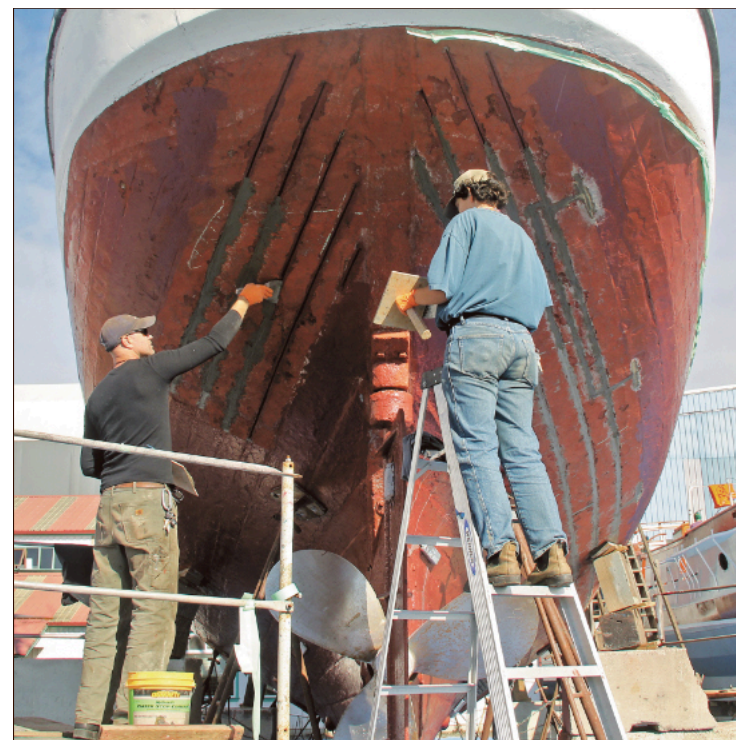
The stern hull of the Polaris has been corked and now gets a layer of sealing cement from James McClurg (left) and Puck Page of the Shipwrights Co-op.
