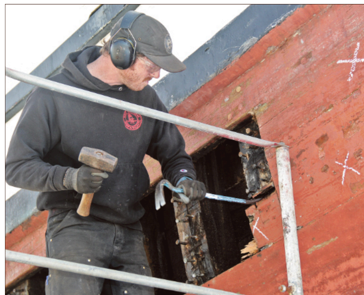
Moses Dane of the Shipwrights Co-op digs out some damaged hull planking near the stern of the Seymour. Some seven Co-op workers are assigned to each schooner.
