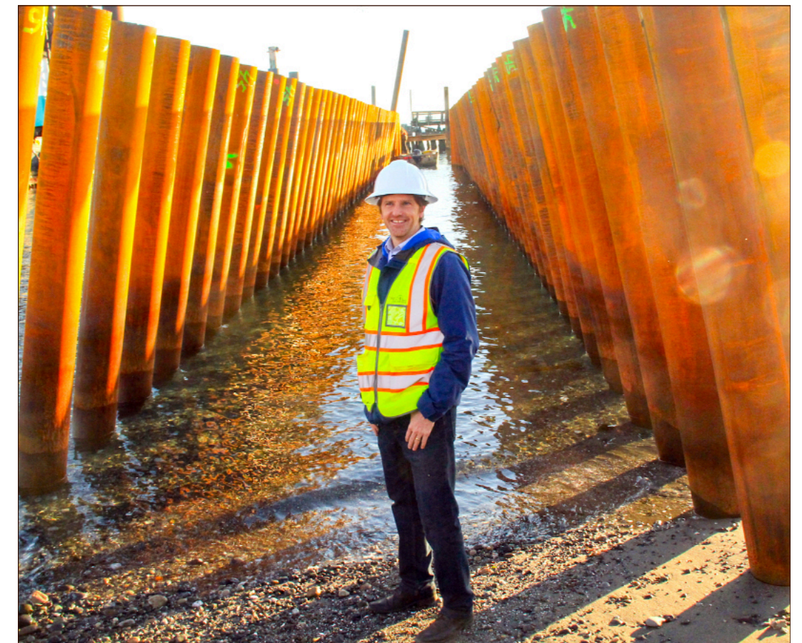
Director of Capital Projects & Port Engineer Matt Klontz stood at low tide beneath the new steel piles driven as part of the jetty rebuild at Point Hudson in early 2023. When the jetties were done, they were about three feet taller than the ones they replaced.
