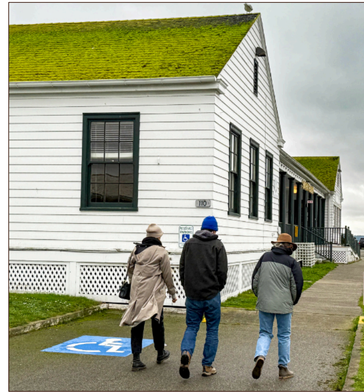
Many of the roofs on Port Hudson’s buildings, put up in 1935, are cement asbestos tiles. The nine buildings that still have these tiles could have them replaced in the future, with the help of the IDD fund.
