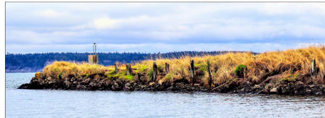
What’s left of pilings originally placed in the mid-1930s are shown in this photo of the entryway into the Boat Haven Marina. This section of the breakwater could be rebuilt, thanks to IDD matching funds.
