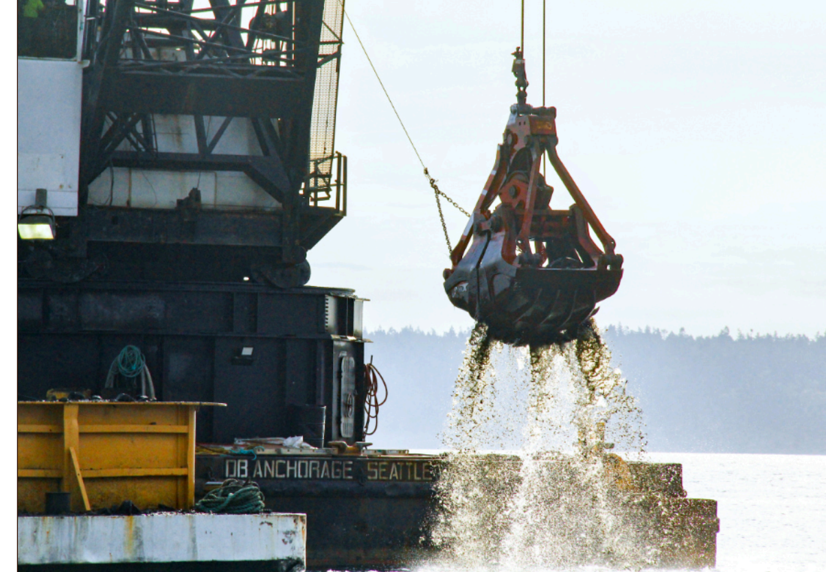
Orion Marine, based in Tacoma, won the contract to tear down the old jetties, and build the new ones with steel pilings and fresh rock. The design is similar, but taller, than the replaced jetties. Orion got the work done on time and under budget.
