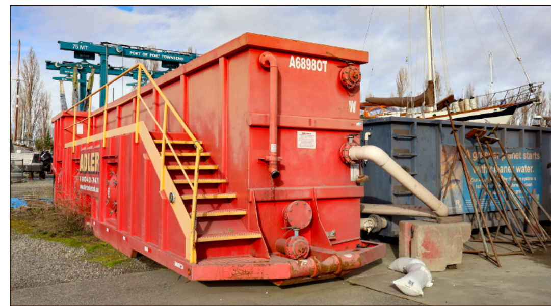
Today's stormwater collection and treatment system in the Boat Haven Boatyard relies on a few treatment components around the boatyard. A newly designed and constructed system would instead bring stormwater to a central filtration system with four successive layers of treatment.
