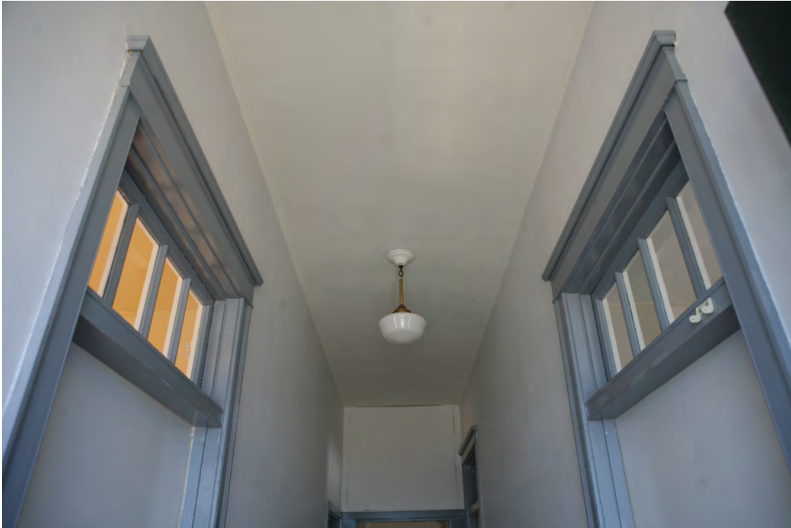
Interior detail view of relites over doorways and trim, Main Building, July 2020.
