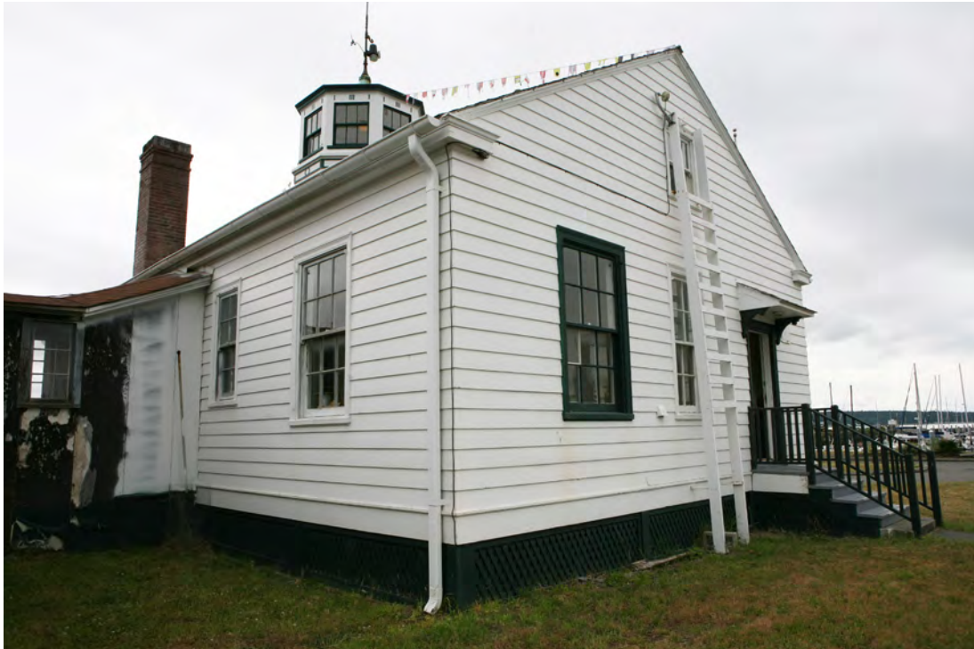
Top: SE corner of Cupola Building, July 2020. Bottom: NW corner of same, July 2020.
