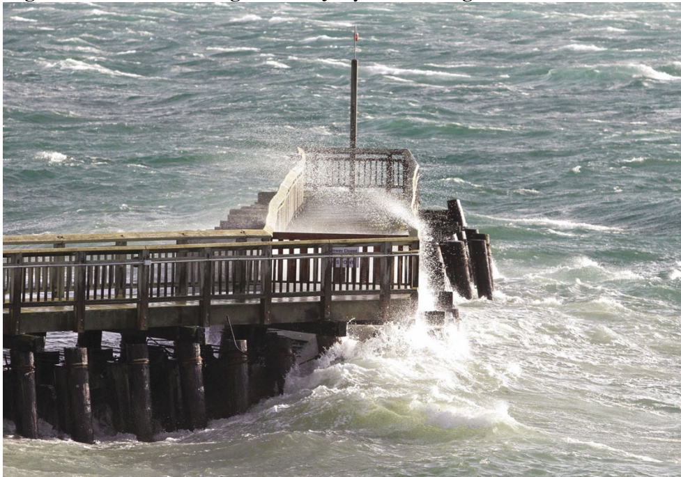
Figure III-7 – Seaward Leg of South Jetty Arm During a December 2018 Storm
