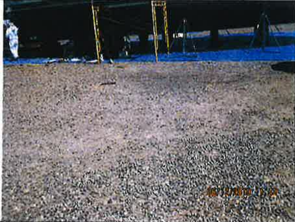
Photo 3 of 6: Storm drains after treatment are sealed preventing new contaminants mixing with the treated stormwater. The facility also removed contaminated soils then filled the areas with washed gravel.
