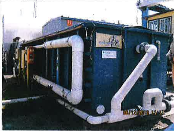
Photo 1 of 6: The boatyard modified their existing stormwater RX system installing Chitosan treatment. The water now flows through the flocculent before being treated in the stormwater RX unit.
