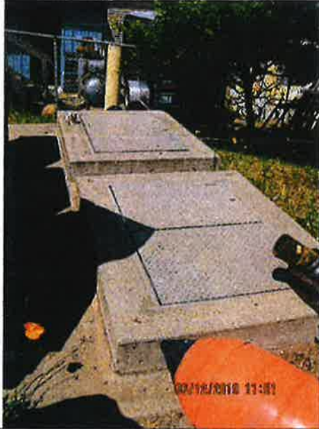
Photo 5 of 6: During lower tides after entering the stormwater system the water flows to the bay. During higher tides it is held in Vault 3. When the vault fills a sump pump turns on then pumps the water to the bay preventing flooding of the boat yard.
