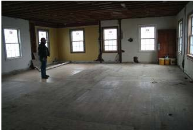
T’s future dining room, with sweeping views of the Sound from the southeast tip of Point Hudson, was formerly partitioned into sleeping quarters for the nurses at the original quarantine station.
