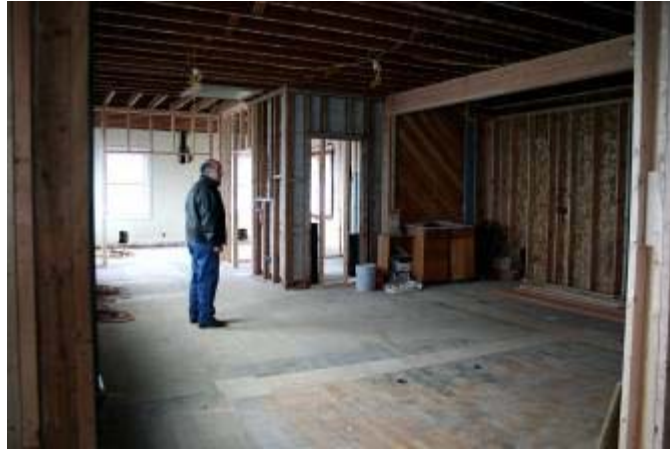
T's new bar and cocktail lounge will be located in the space created by enclosing a porch (the alcove pictured at right).
