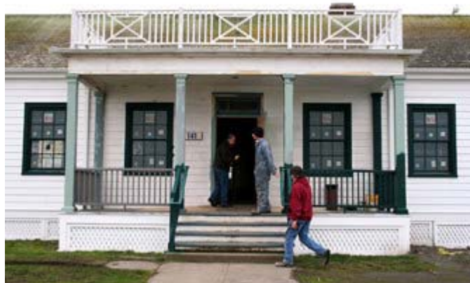
A railing above the portico that had been removed in the 1940s has been rebuilt to its original specifications.
