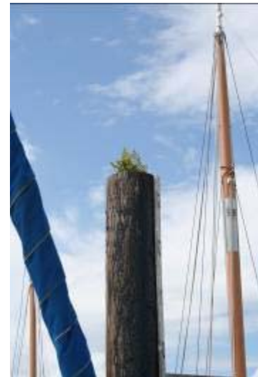
Rotten pilings grow vegetation
