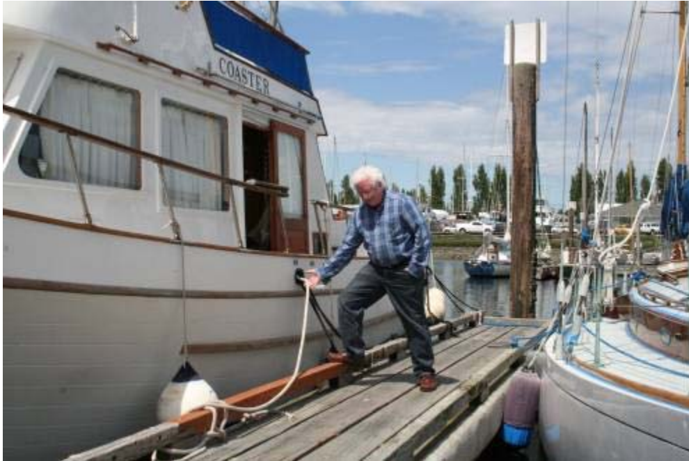
Moorage tenant Stephen Lewis shows the section of bull rail that failed (and was replaced) at his A/B Dock slip
